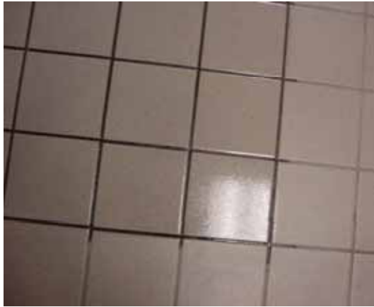
Glazed Tile Bathroom Winn Dixie Distribution Center
